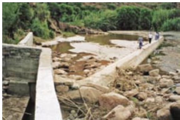
Photo 2.3 Intake in San Roque-Capellania irrigation system
