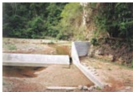
Photo 2.5 Intake in Caigua irrigation system
