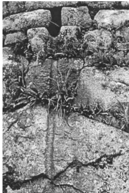
Figure 10. Engineers Strategically Placed 129 Surface Drainage Outlets in Walls to Drain Interior Ground Surfaces. This Drainage Outlet Was Fitted with Vertical Channel to Avoid Splash.
