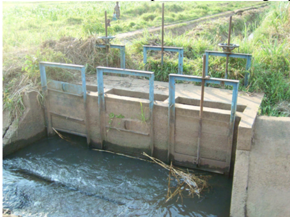
Photo 5.1: Dilapidated gates on main canal missing wheels
